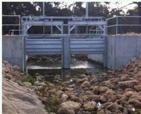
Figure 39. The adjustable height weir, receiving flows diverted from the Mealup Main Drain. Photo – H Bucktin/DEC.
