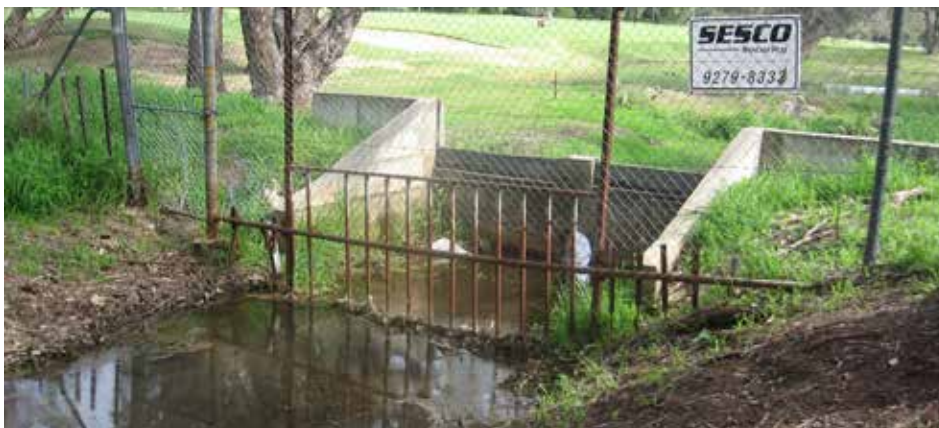
Figure 48. Structures to prevent litter and debris from entering drains and wetlands need to be cleared regularly. Photo – DEC.
