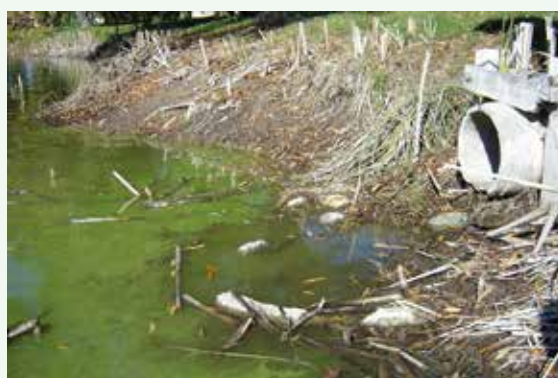
Figure 24. This stormwater drain transports nutrient rich water into the lake, contributing to the bloom pictured here. Photo - D Mort/City of Rockingham.
