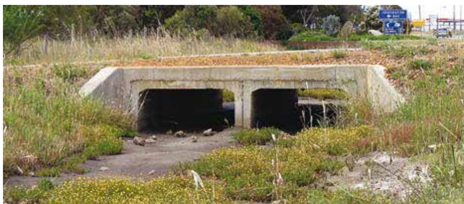
Figure 14. Culverts can enable some degree of water flow beneath barriers such as roads, but they need to be well designed in order to avoid problems such as erosion and sedimentation. Image – Department of Water.
