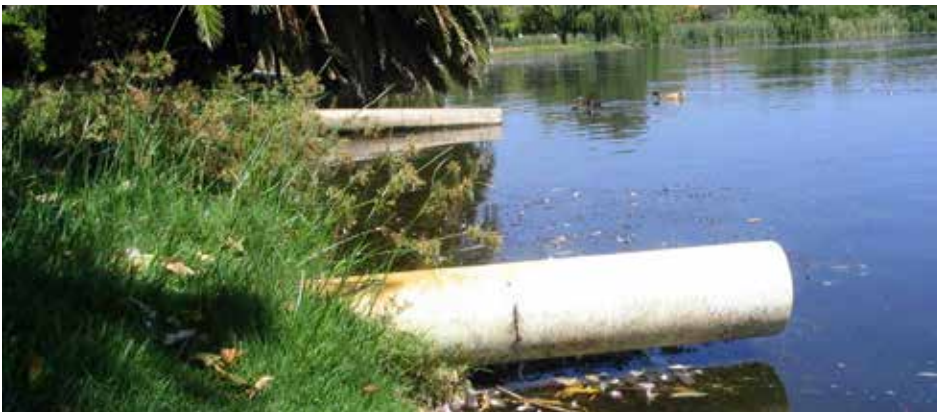
Figure 10. Pipes discharge stormwater directly into Lake Monger, Perth. Photo – L Mazzella/ Department of Water.
