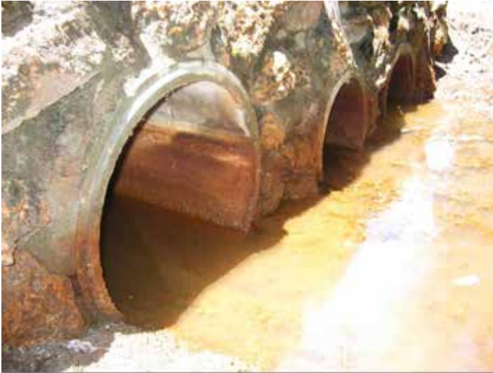
Figure 37. Road culverts that have corroded as a result of acidic drainage. Photo – B Degens/ Department of Water.
