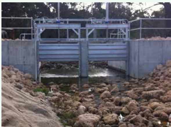
Figure 40. The adjustable height weir, receiving flows diverted from the Mealup Main Drain. Photo – H Bucktin/DEC.
