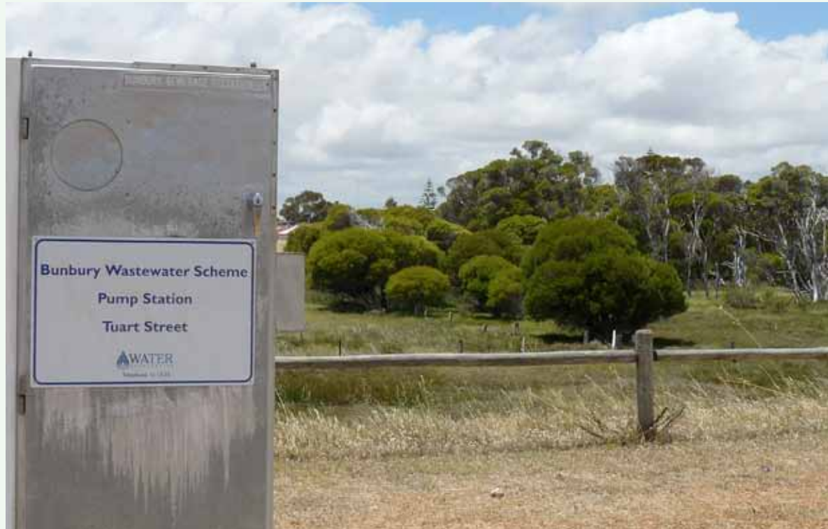
Figure 5. A pumping station. Photo – C Mykytiuk/DEC
