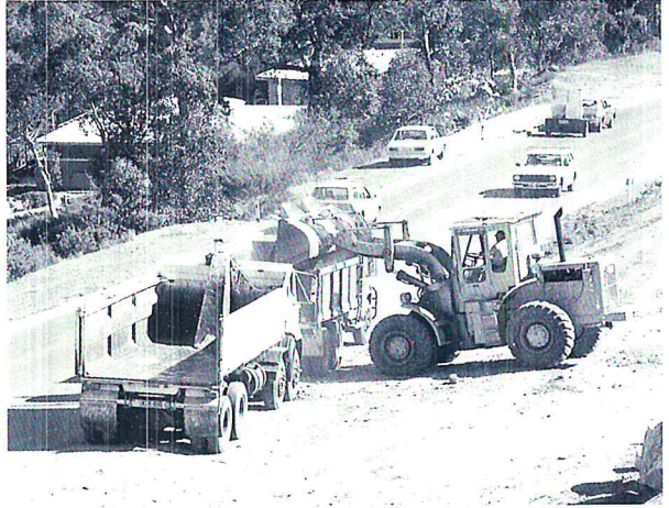
Noise and vibration from road construction and maintenance activity can be a nuisance and cause damage to buildings. (Photo MRWA)
