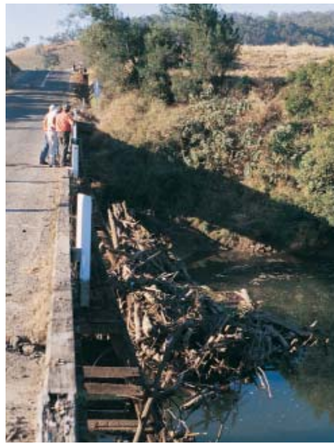
Woody debris trapped against a bridge on the Mary River, SE Qld. Photo Ian Rutherford.
