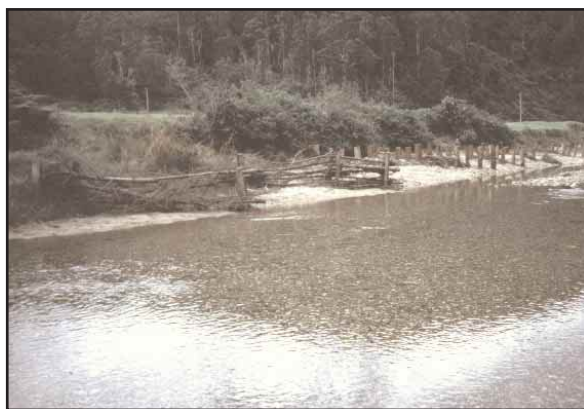
Figure 15. Pin retards and brush retards used to stop bank erosion and stabilise an artificial bench on Taylors Arm, a tributary of the Nambucca River, in northern New South Wales.
