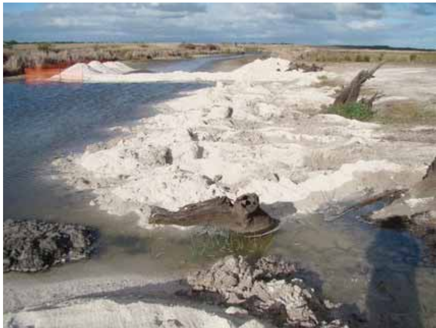
Treating acidification with limestone, Finnis River, Lower Murray Lakes, SA (© DEPARTMENT FOR ENVIRONMENT AND NATURAL RESOURCES SA)
