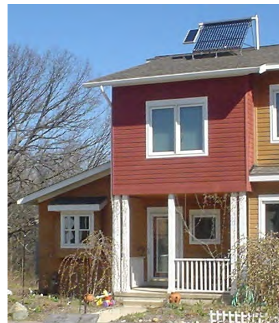
Figure 30.2. A solar water heater providing hot water for a family in Michigan. The system's pump is powered by the small photovoltaic panel on the left.
