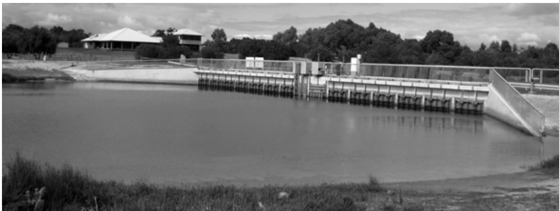
Flood gates in the Vasse–Wonnerup Ramsar site. Photo – Kym Pearce (DPaW)
