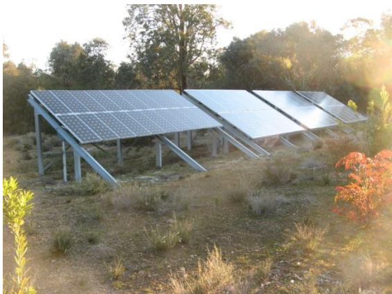
Figure 8: Current Solar Array (Photo: Elise Pinto, 2011)
