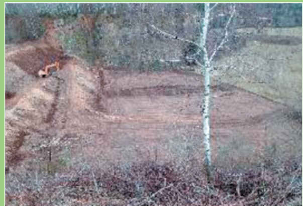
Soil stripping and vegetation clearance being undertaken in winter, outside the bird nesting season
