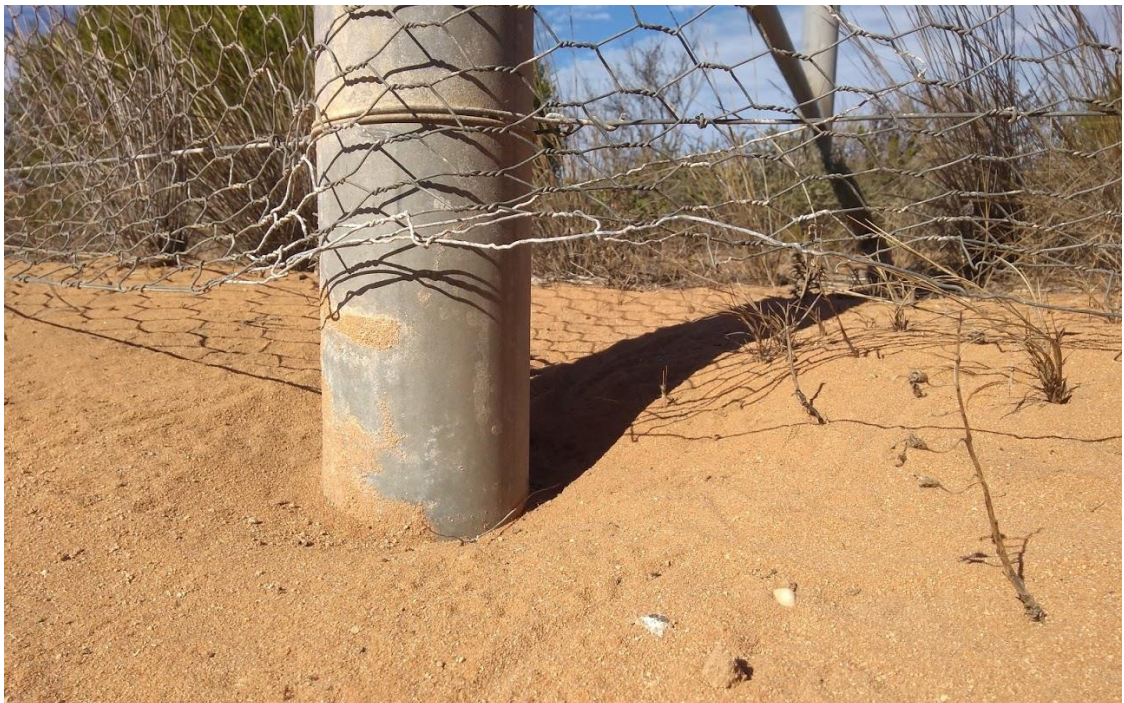
Figure 16. Image of hole in management fence, 500m west of main gate (25/05/2019) (© S. Cowen/DBCA).
