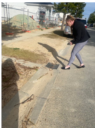
Left: Sand drift into nearby drain at residential building site, Chelydra Point, North Coogee, City of Cockburn.
