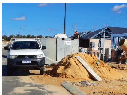
Left: Builders sand partially dumped on the road by sand carriers at building site on Windich Rd, Mandogalup; another new subdivision in the City of Kwinana. (Photo credit: Bronwyn Scallan)
