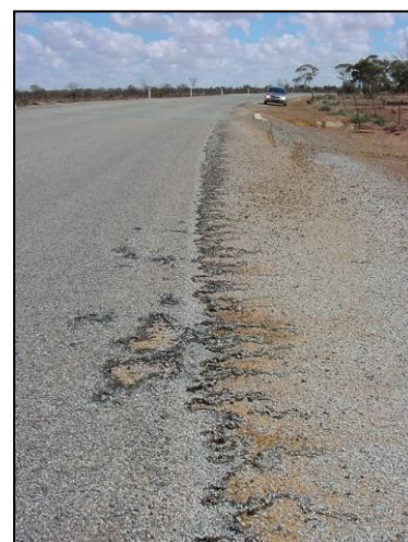
Salt damaged road surface
