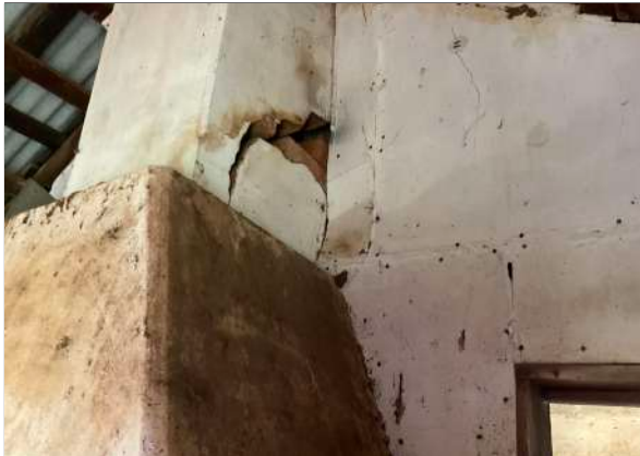
Damage to brick chimney
