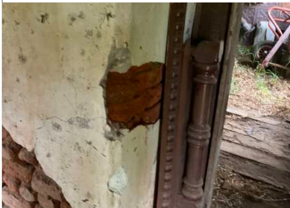
Damaged timber detailing to door frame
