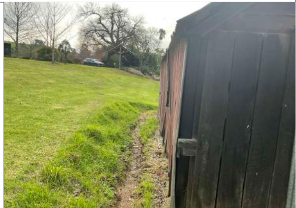
South west corner with missing timber board
