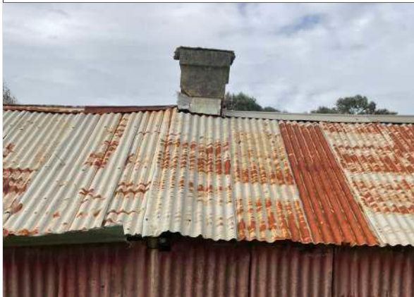
Rusted roof sheets and chimney
