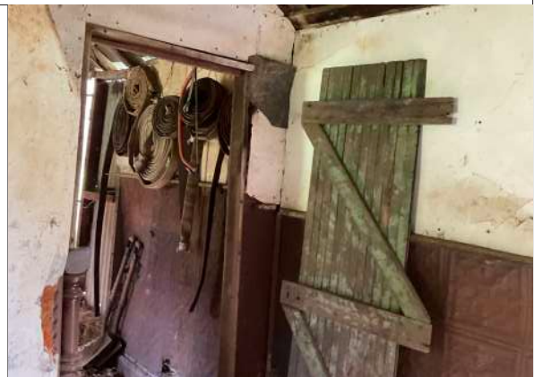
Internal door damaged and removed
