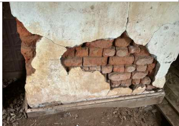
Damage to render at base of chimney
