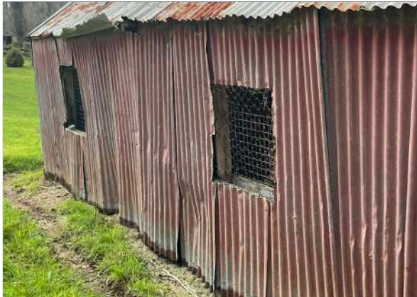
Window and damaged steel sheets along western elevation
