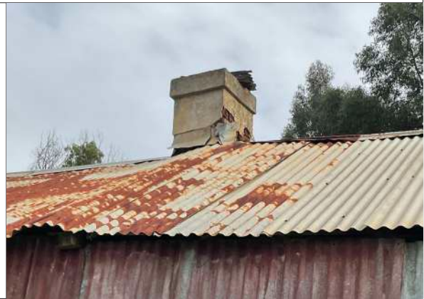
Damaged render to chimney
