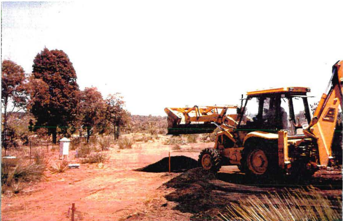
Photo 6: Trial excavation at Site C “wet”. Note the low levels of dust generated.
