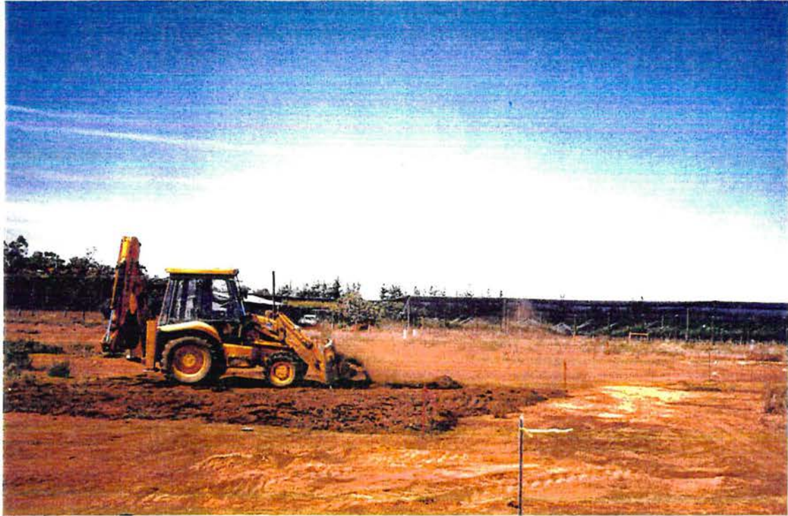
Photo 1: Excavation of Site A "wet". Note the dust generated due to disturbance of the dry underlying soil
