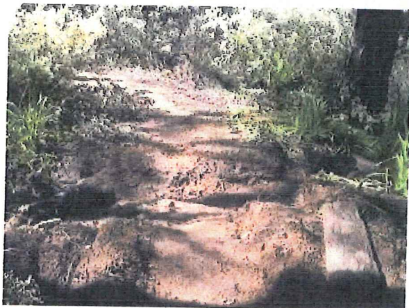
Figure 12: Localised erosion downstream of Mundaring Weir Road.
