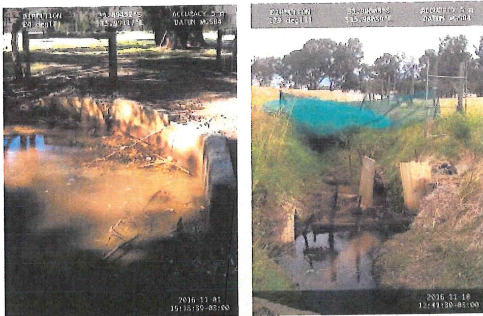
Figure 51: Stagnant water in northern alignment of the Helena River in Woodbridge. Figure 52: Damaged golf course fencing in drain from Rosehill Estate.
