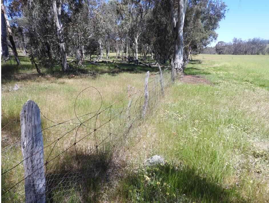
Photo 21: Damaged fences along the western boundary in the Northern Section of the reserve
