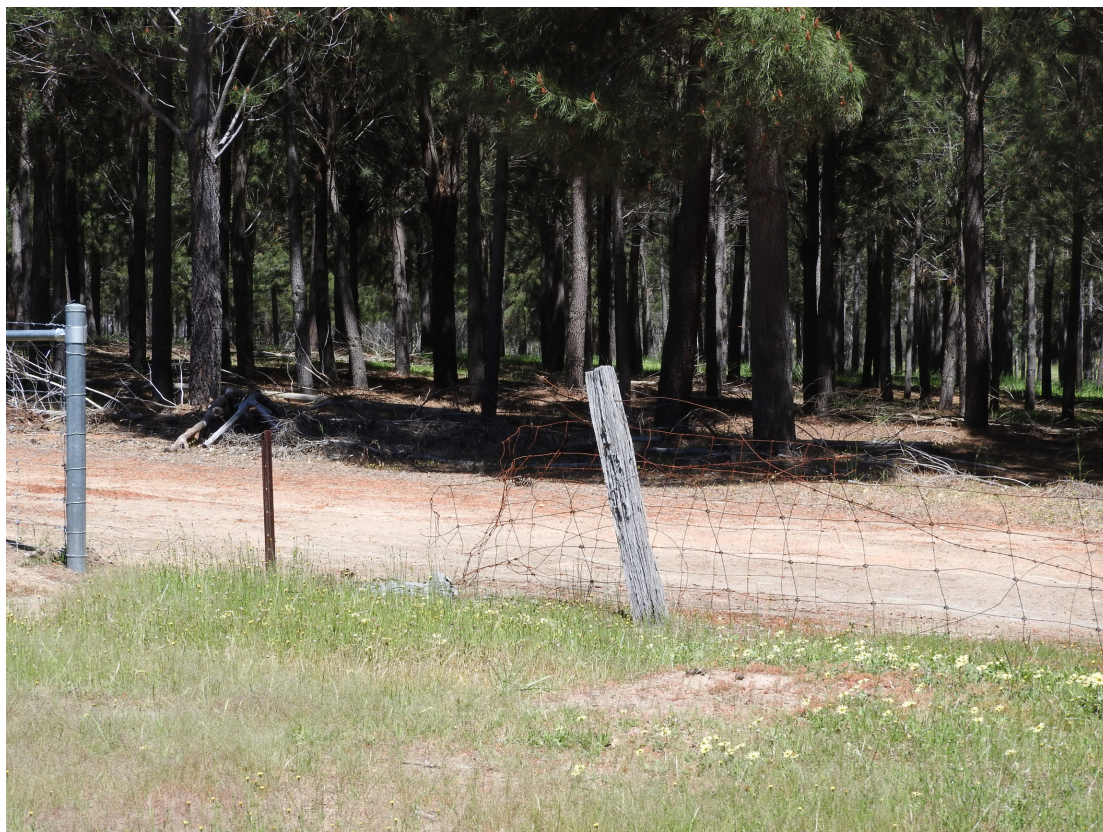
Photo 19: Damaged fences along the western boundary of the Southern Section of the reserve
