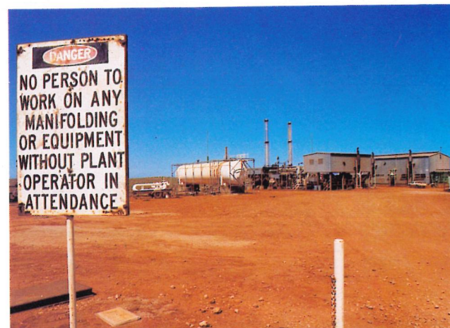
LPG plant and compressor station
