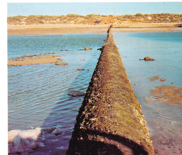
Submarine pipeline at low tide
