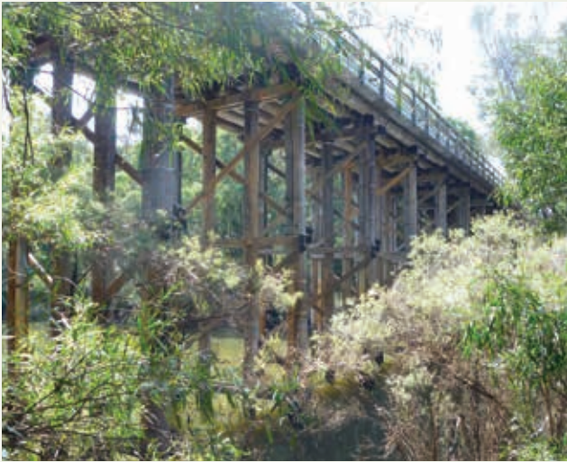
Sues Bridge area. The height of the bridge illustrates the depth of the valley and height of expected floodwaters October 2010. A. Brearley.
