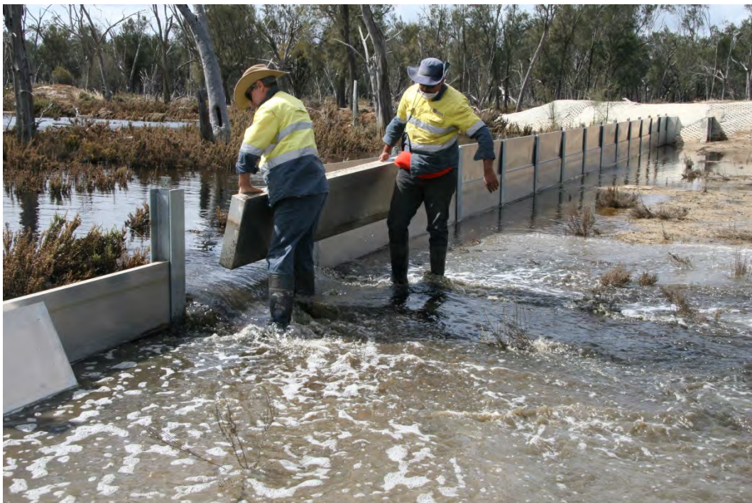
Opening of diversion gates at Toolibin Lake
