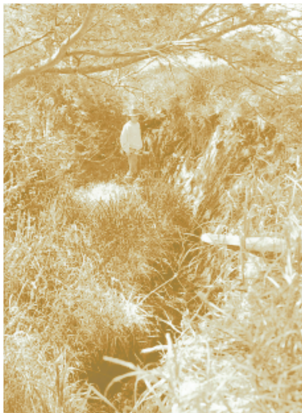
Deep seated rotational failure, Latrobe River, Victoria. Photo by Ian Rutherford.
