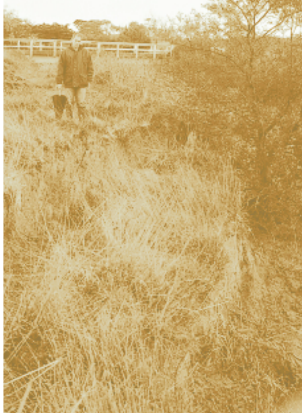
Slab failure in the Tarwin River, Victoria. Photo by Ian Rutherford.
