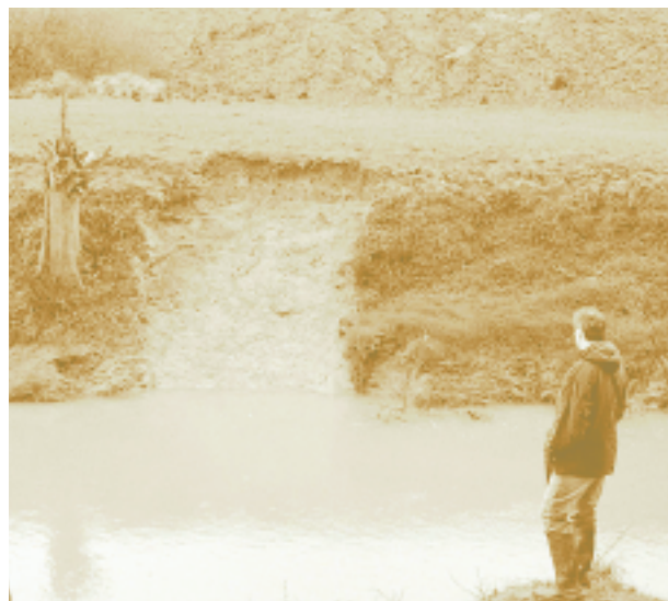
Shallow slip failures on the Tarwin River, Victoria. Photo by Ian Rutherford.
