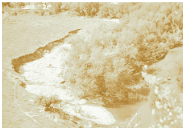
Willows in the Torrens River, South Australia, divert flow around them and erode the banks. Photo by Ian Rutherford.
