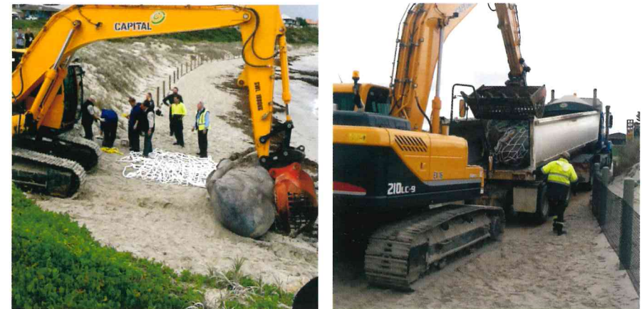
Left: Beach side before securing the whale carcass. Right: Placing the secured carcass in a truck for disposal.
