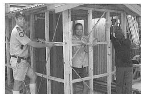
(L-R) Greenough Regional Prison Officer Shaun Tormey and TAFE Construction Lecturer Matt Silvester help prisoners disassemble a Dinkum Dunny for transport to Stockyard Gully.
