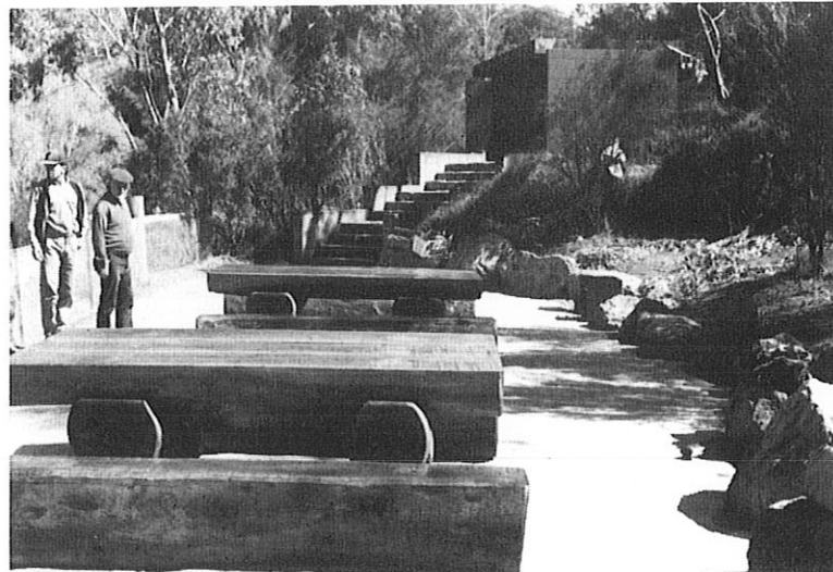
Figure 7 Completed tables. Refurbished ablution block in background. Edge of site on right hand side has been edged with rock for retention of the bank and to provide seating.
