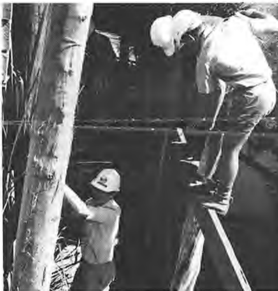
SECOND-year cadets construct the boardwalk beneath the bridge at One Tree Bridge recreation site.
