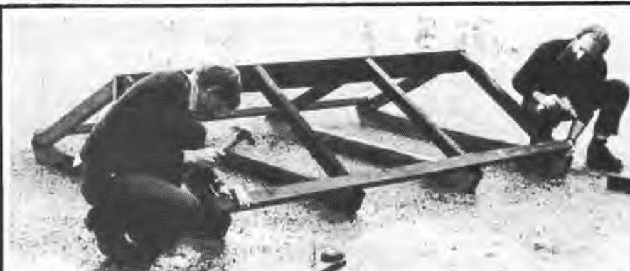
GEOFF and Mark build an information bay at the start of a heritage trail on Stony Hill in Torndirrup National Park.
