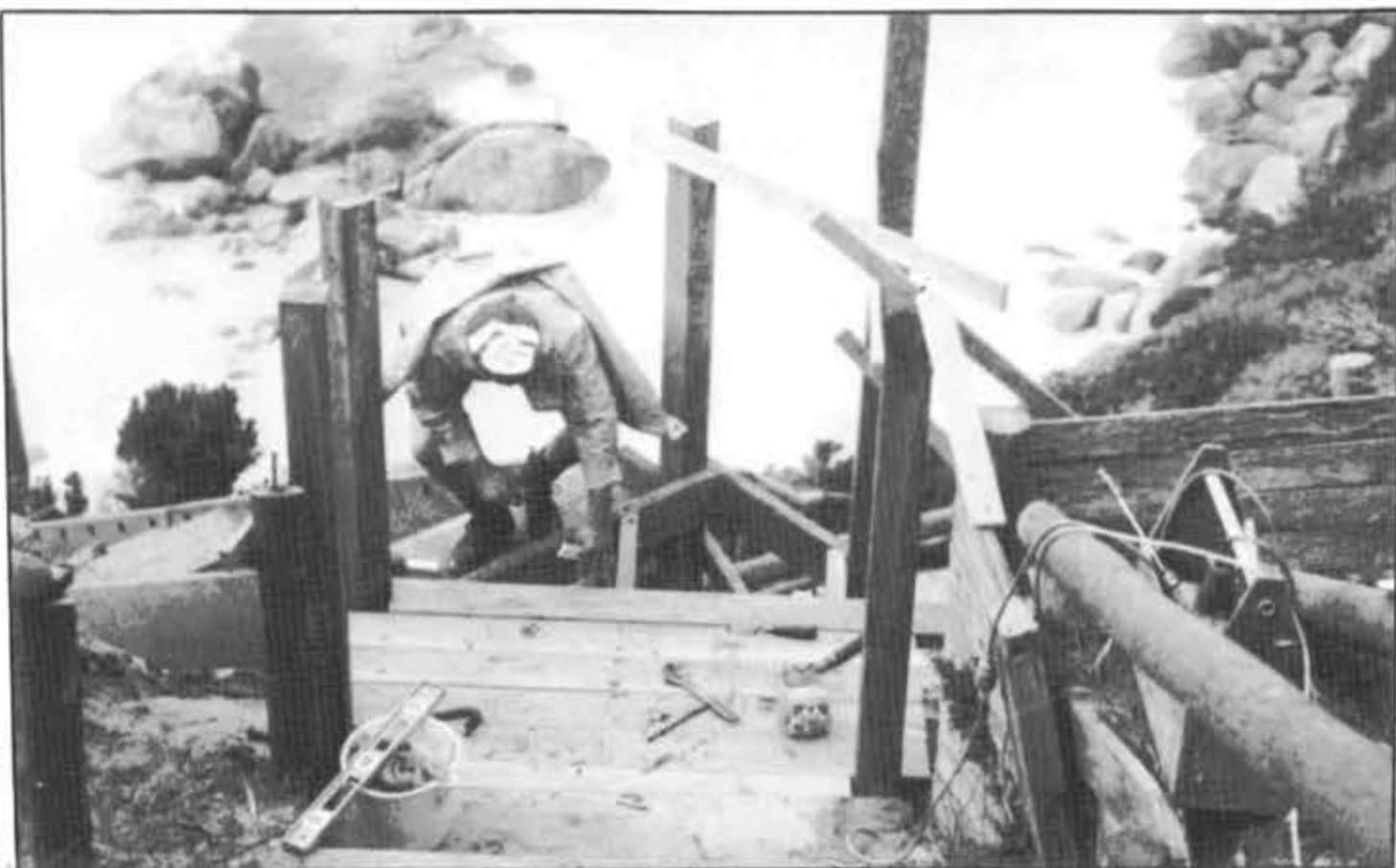
Contractor Reg Eastough working on the steps' first landing, some 80 metres above the beach.
