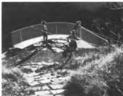
Sections of the safety railing being fitted on-site at Joffre Gorge in the Karijini National Park.
