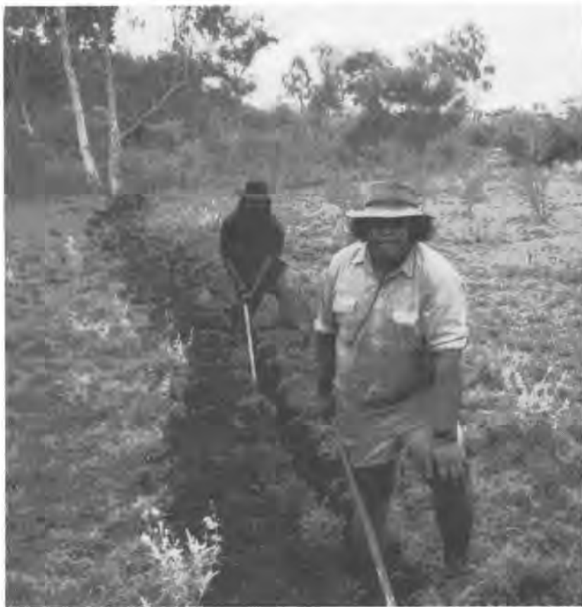
Peter Limerick (rear) and Damien Walker prepare to lay waterpipes to car park development. Photo by Russell Bone
