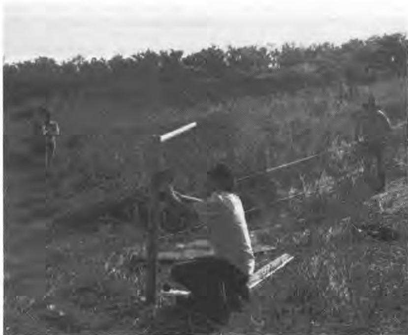
CALM workers erecting the fence around a remnant rainforest patch at Mitchell Plateau
