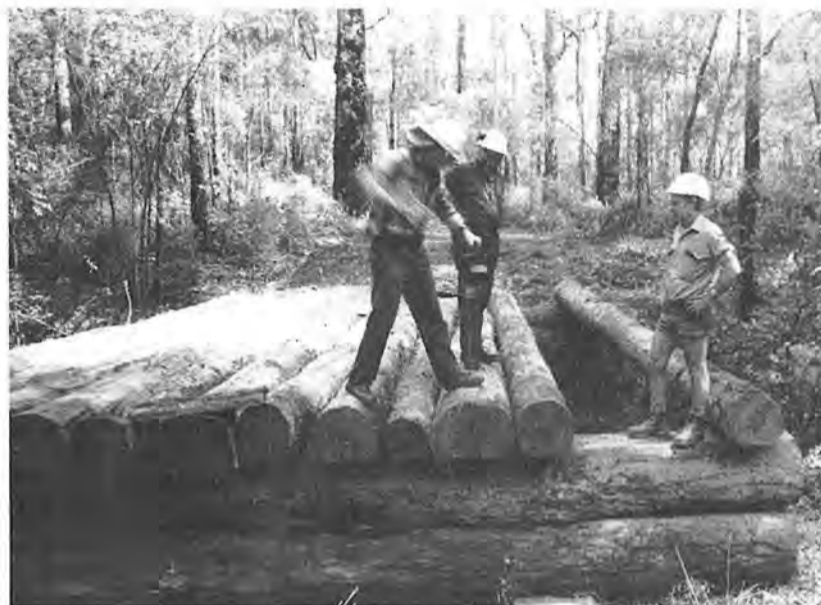
Collie forester Glyn Yates demonstrates use of equipment on-site at a new bridge being built at Honeymoon Pool to new campsites.
