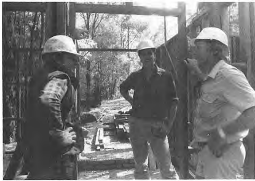
Inspecting progress on a new toilet block at Honeymoon Pool are (left) Collie reserves officer Rob Brazell, Collie senior forester Alan Hordacre and Bunbury parks and reserves officer Neil Taylor.
