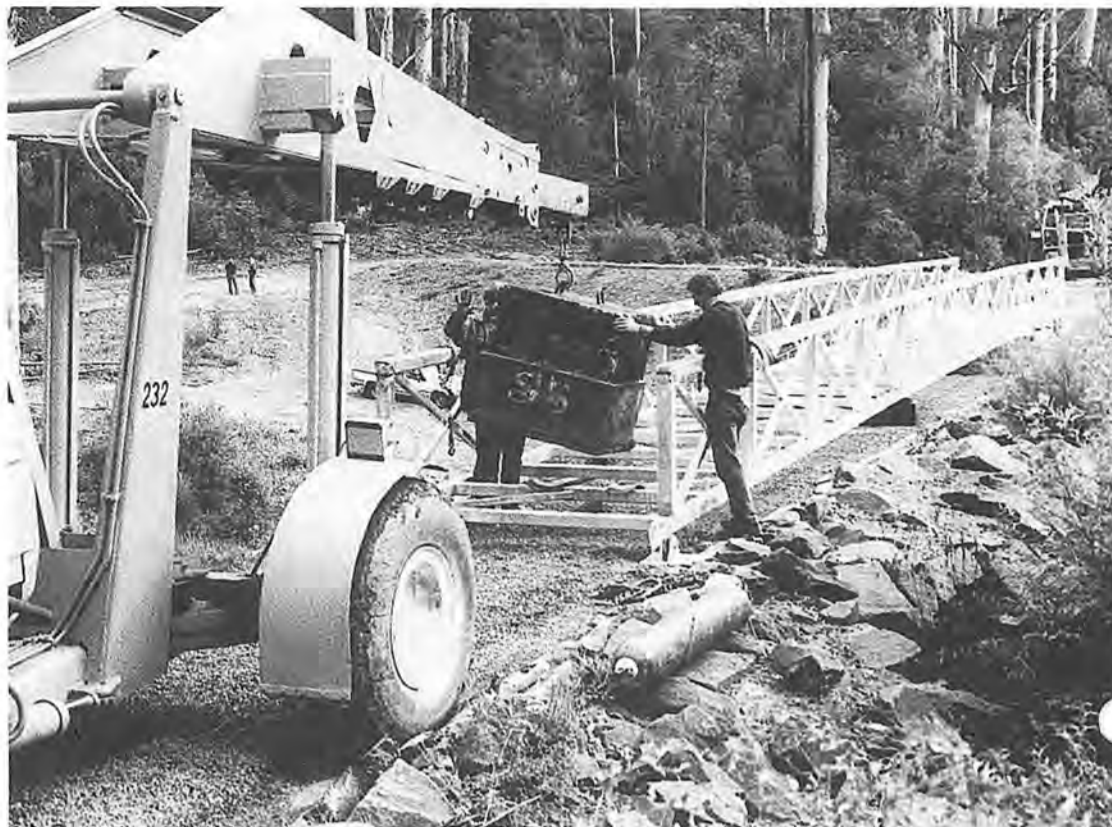
With a crane at either end, the bridge is manoeuvred into position. Photo by John Neal
