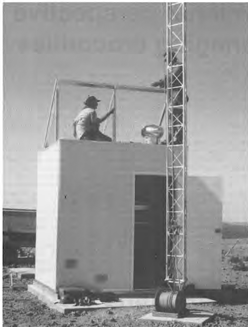
Operations officer Russell Bone helps radio communication officer Max Speer (hiding behind the tower) to assemble brackets for the solar panels which power the radio equipment. Photo by Graeme Hutchinson
