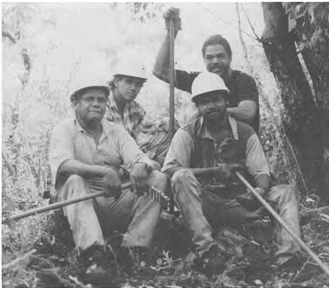
Left to right Vince, Francis, Harry and Franklin take a welcome rest from some back-breaking work during the walk trail construction. Photo by Murray Banks
