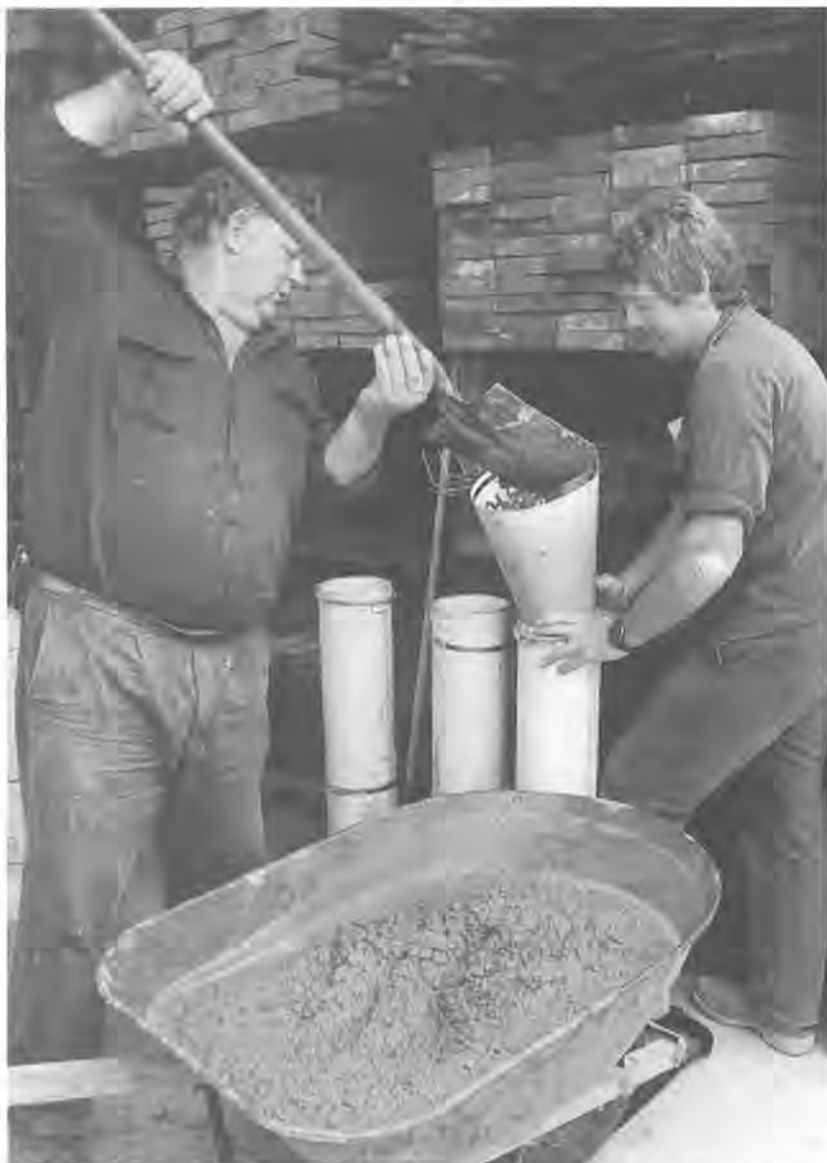
Allen Clarke, right, holds the funnel steady while Keith Harris loads one of the bollard moulds — a new idea aimed at stemming the cost of vandalism. Photo by Tammie Reid
