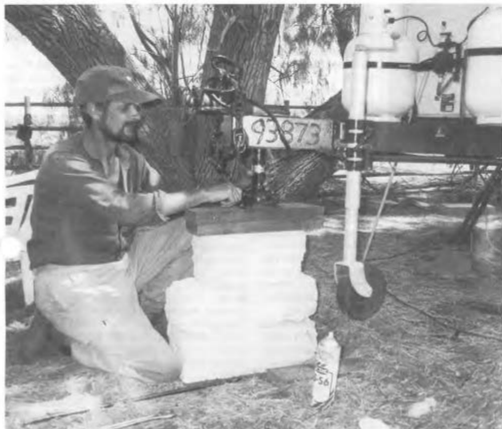
Ray Smith levels the caravan before constructing the annexe that will be the Project Eden Control Centre.
