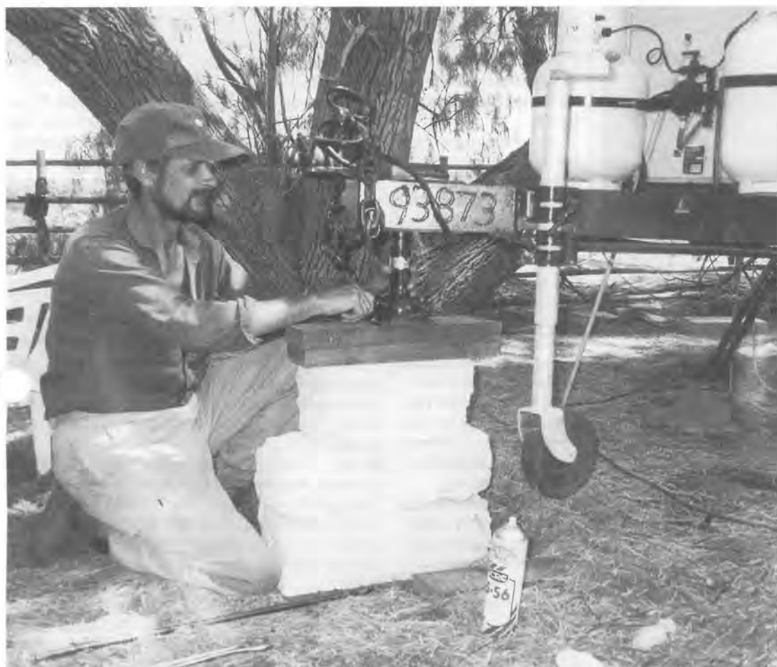
Ray Smith levels the caravan before constructing the annexe that will be the Project Eden Control Centre. Photo by David Gough
