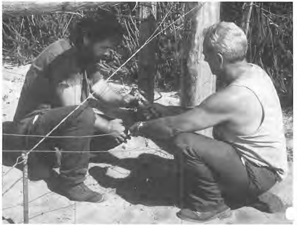
CALM Perth District staff, Neil Osman (right) and Julian Morris putting finishing touches on the fence that will protect the tumulus springs from grazing and trampling by cattle. Other Perth District staff construction and maintenance worker Wayne Calvert also helped with the fencing and forest ranger Ken Borland and reserves officer Rod Martyn did the planning for the operation.
