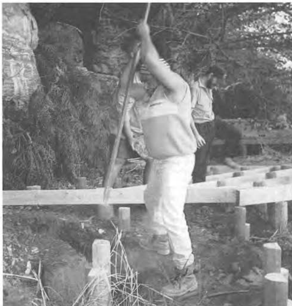
Laying down stumps and bearers for the boardwalk and viewing platform at Fern Pool are, left to right, Adrian Lawson, CEPANCRM leading hand Phil Young, and Joseph Limerick. Photo by Johnny Parker
