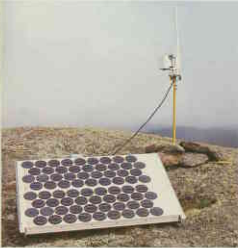
▲ A solar bank (front) provides 24-volt power to batteries which operate the transponder (rear) on top of Mt. Roe.
