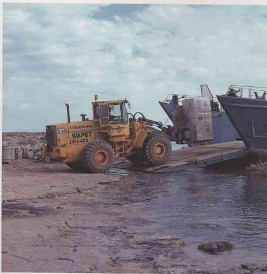
Barge Karinyah II , supplied by West Australian Petroleum (WAPET), unloading at Hermite Island. Photo – Andrew Burbidge
