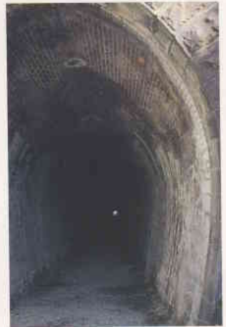
Top: A major accident occurred in the park in November 1942, when locomotive crews passed out from heat and fumes in the poorly ventilated tunnel. Photo – Trevor Marshall
