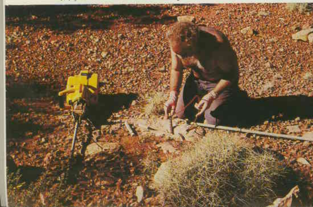
▼ In some exceptional cases the ground defied even a rock drill and small charges of explosive were needed to break enough rock to set a trap. — Photo J. Lane.
