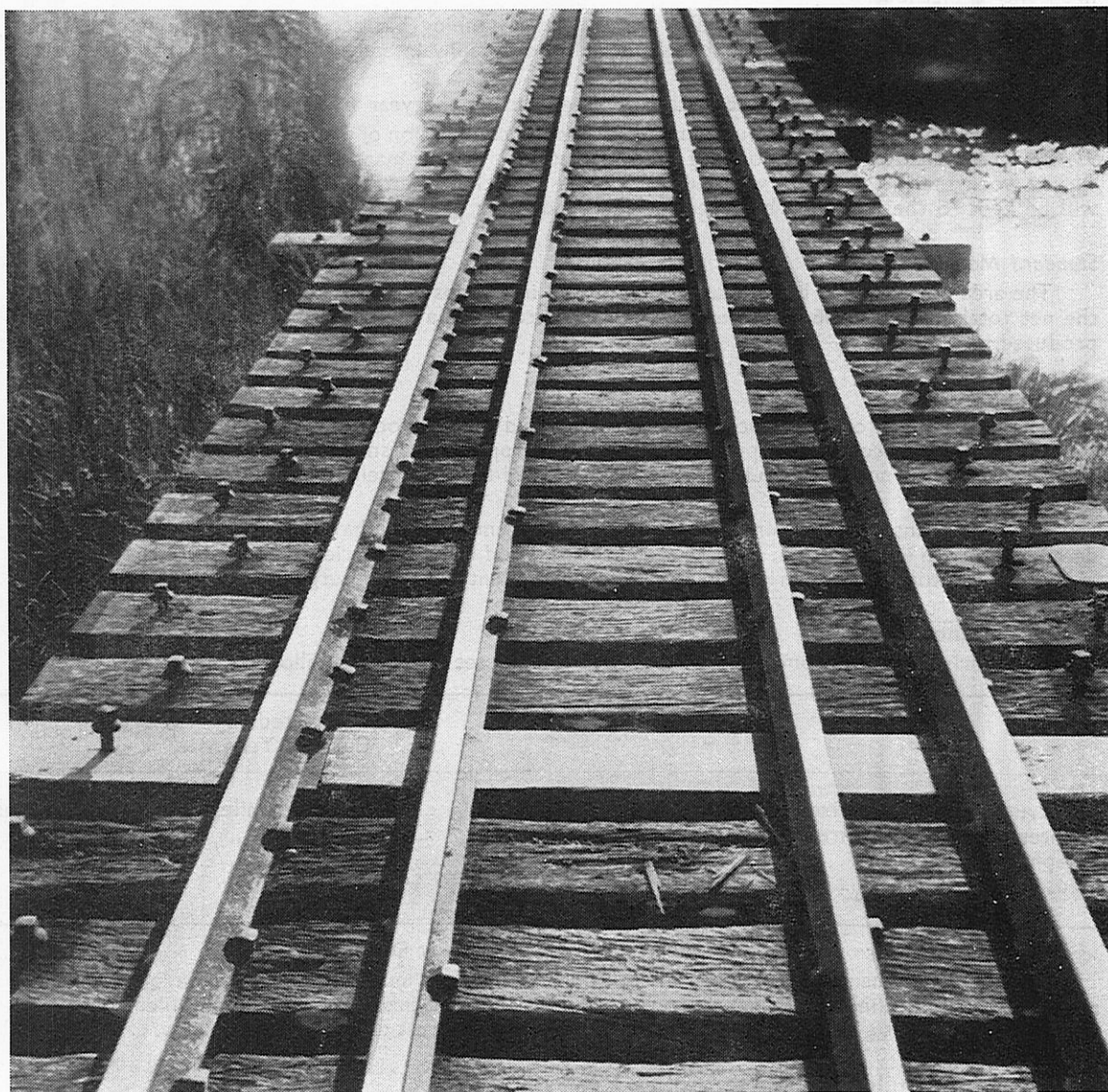
Jarrah sleepers on a bridge in Otago Province, New Zealand. After 50 years of service, only two of the original 200 sleepers had to be replaced. The dog spikes are still holding firmly in the original holes into which they were driven in 1911
