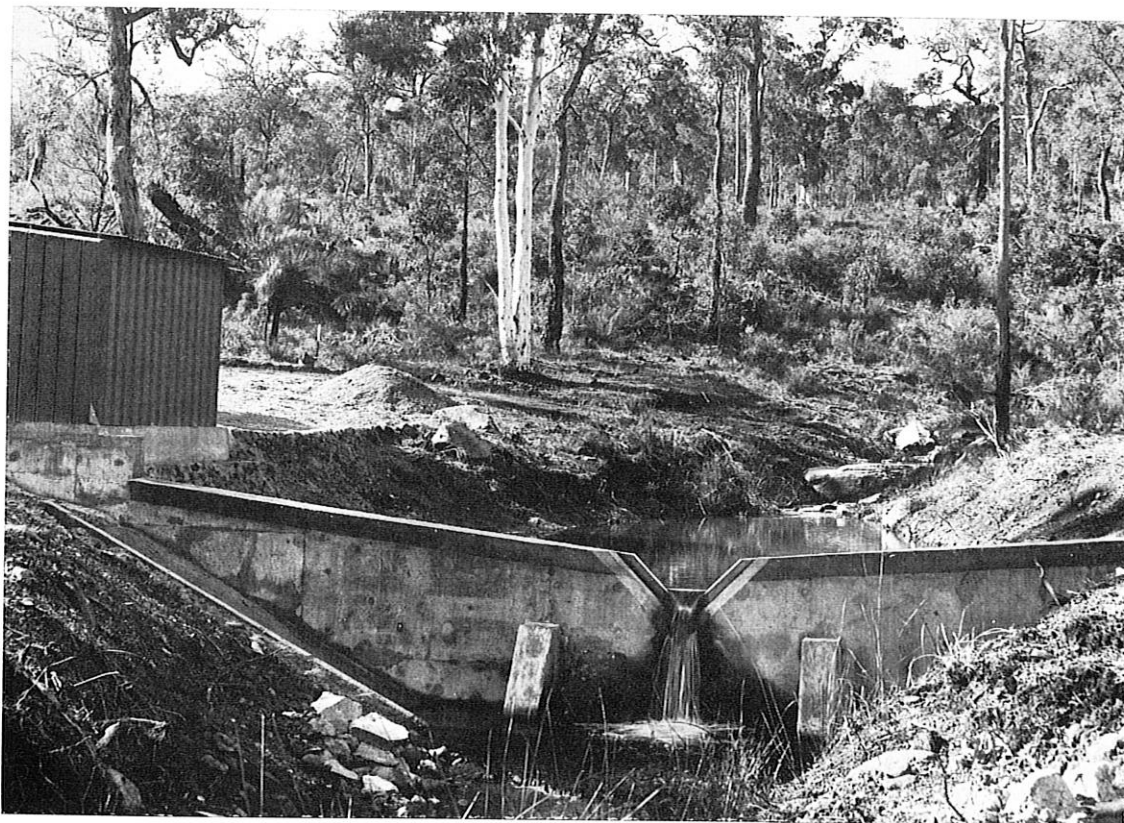
Combination V-notch weir located on a tributary of Marrinup Brook, West of Dwellingup. This is one of seven weirs designed to provide information on the potential to increase water yield in the high-rainfall zone of the northern jarrah forest. The weirs were designed by the P.W.D. Water Resources Section and were constructed by Forests Department personnel.
