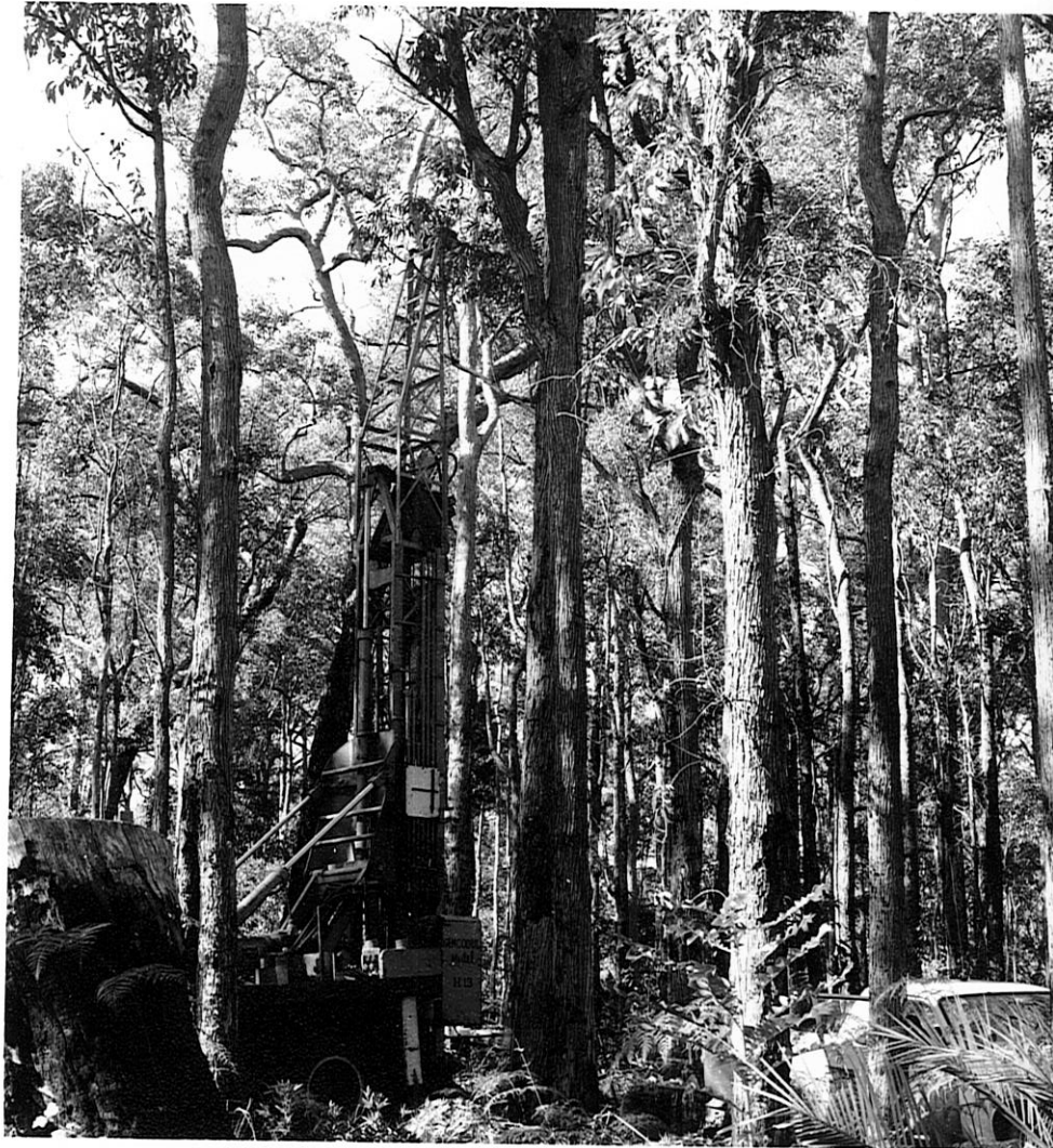
Fig. 4 Drilling rig used to obtain cores for de- termination of salt profile.
