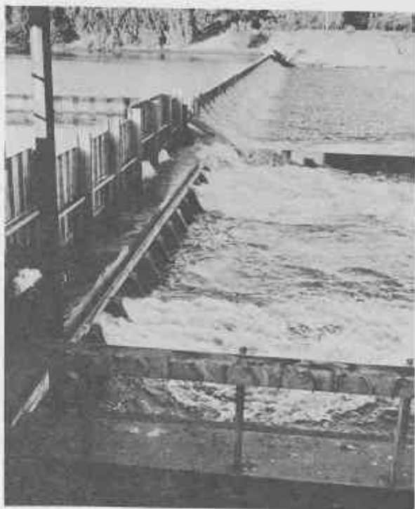
Photo. 3. Fitzroy Barrage - Submerged Outlets in Foreground (L.H.S.) Open
