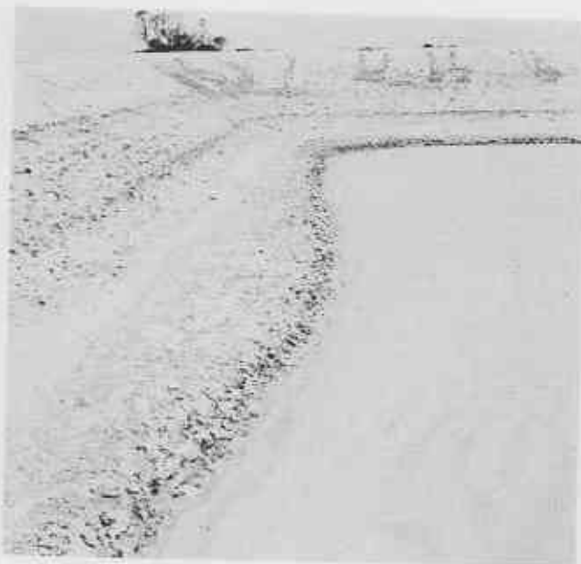
Shoreline and Milky Turbid Water in Carpenter's White, Pipe-clay Dam.
