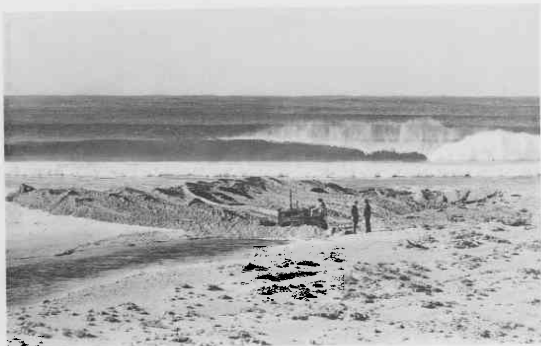
Plate 2—The second half of the channel is bulldozed early on the opening day. A small section of the sand bar, midway along the channel is left unbroken.
