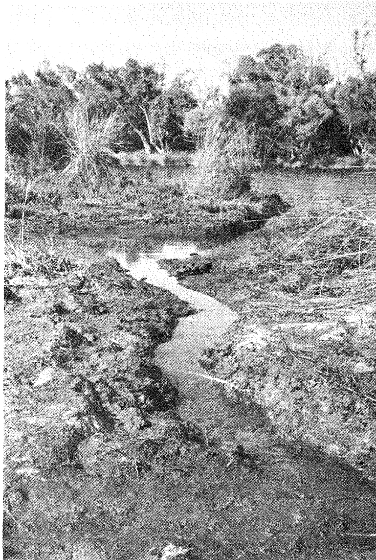
Plate 1 . A very shallow hand-dug runnel (5-10cm) deep connecting a small area of low marsh to a waterway . Such a channel is essentially a formalised natural drainage line. One of an existing set of wheel ruts may be formalised in the same way.
